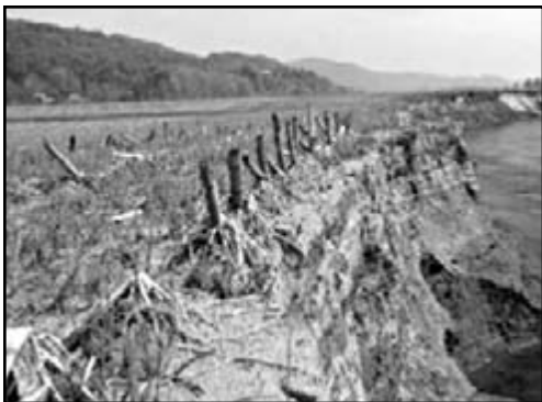
Fast waters caused excessive erosion at this site, which destroyed the stream bank and altered the shape of the land. Roots of plants in a healthy riparian zone prevent this type of damage by slowing water, holding soil, and shielding the bank from the force of rushing water. Photo courtesy of Natural Resources Conservation Service
